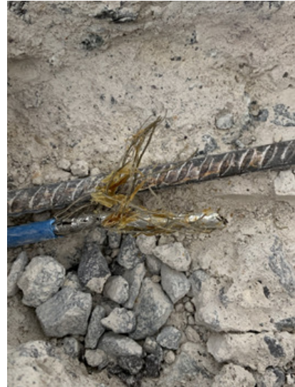
Figure 6. Creation of wax as a result of lightning strike damage.
