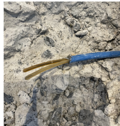
Figure 2. Colour difference after damage to heating wires.
