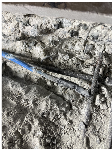
Figure 3. End junction failure.
